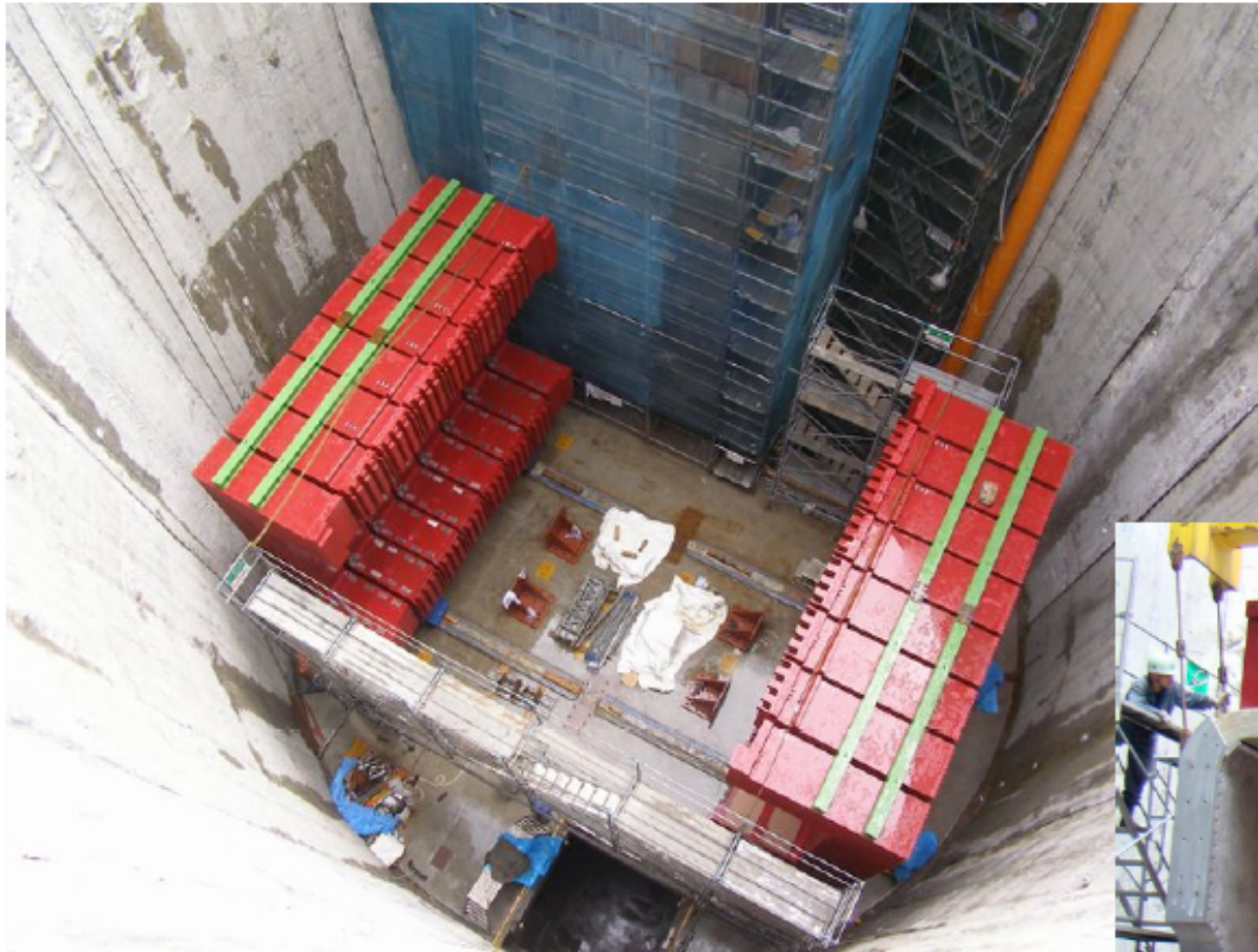
Yokes installation (open position)
